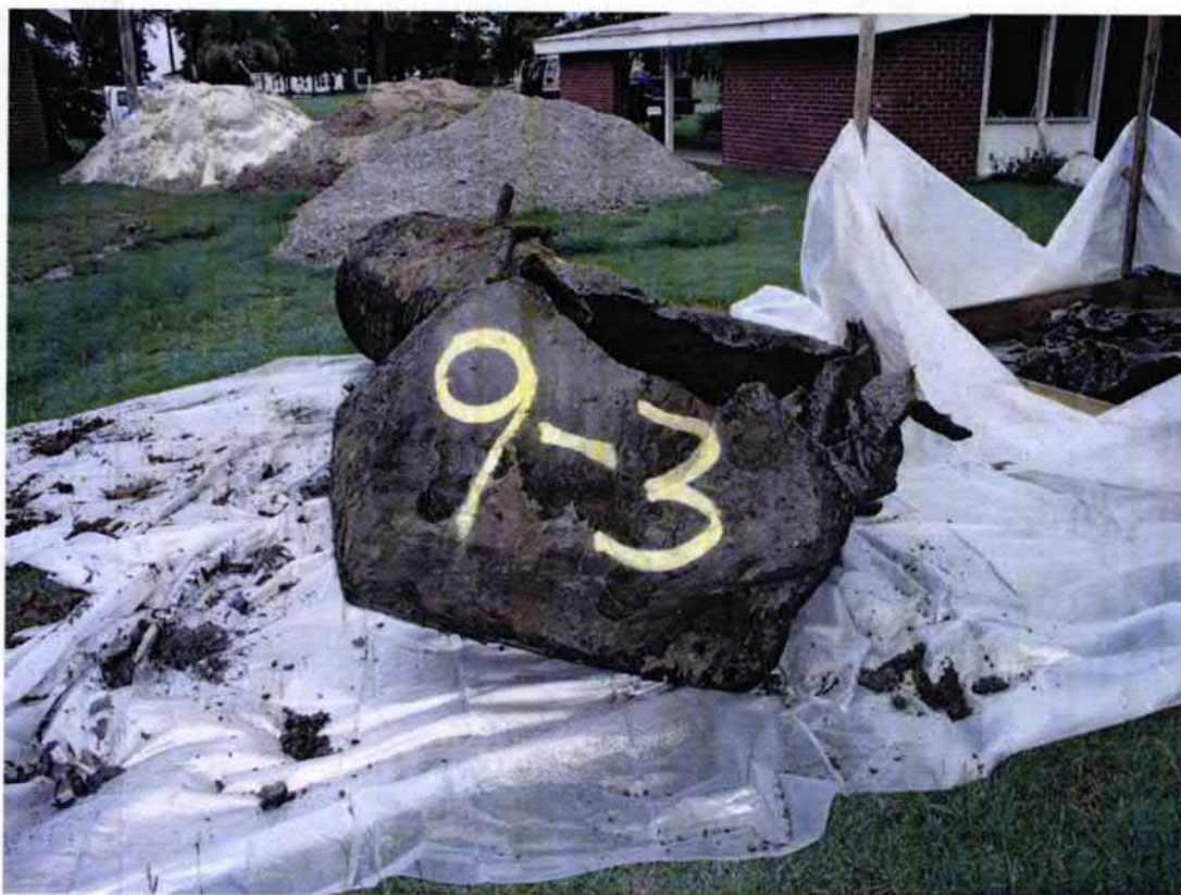
Laurel Bay # 9 / Tank # 9-3.
